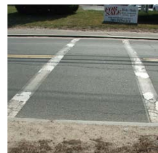
Crosswalk without curb cut ramp
