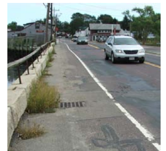
Uneven roadway surface
