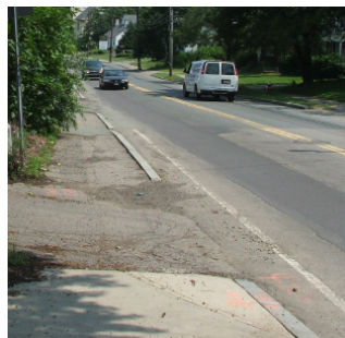
Some of the sidewalks near the study boundary are in need of repair.
