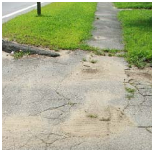
Some sidewalks are narrow and uneven.
