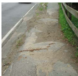
Sand and debris create an uneven sidewalk surface.
