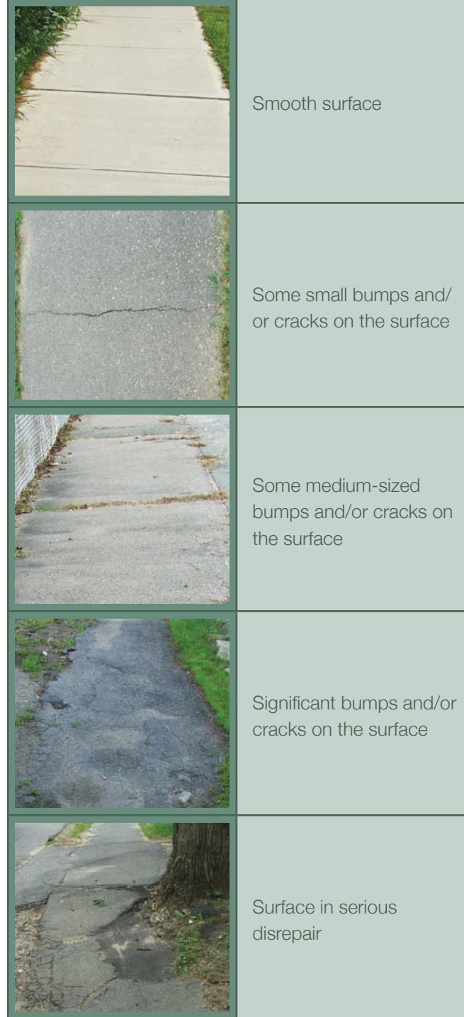
Figure 2 SIDEWALK SURFACE CONDITION SCALE
