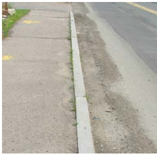
The roadway edges near the study boundary are uneven and contain debris.
