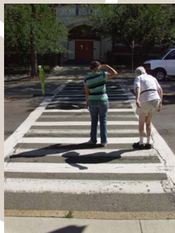
Lack of curb ramps and curb extensions
