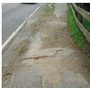
Sand and debris create an uneven sidewalk surface.
