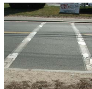
Crosswalk without curb cut ramp
