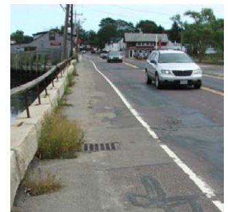
Uneven roadway surface
