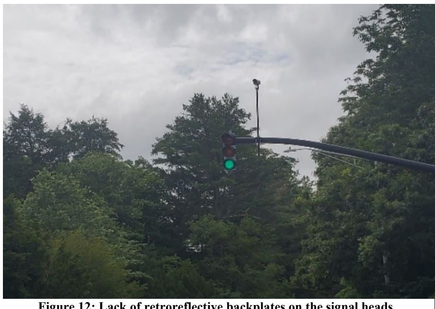
Figure 12: Lack of retroreflective backplates on the signal heads
