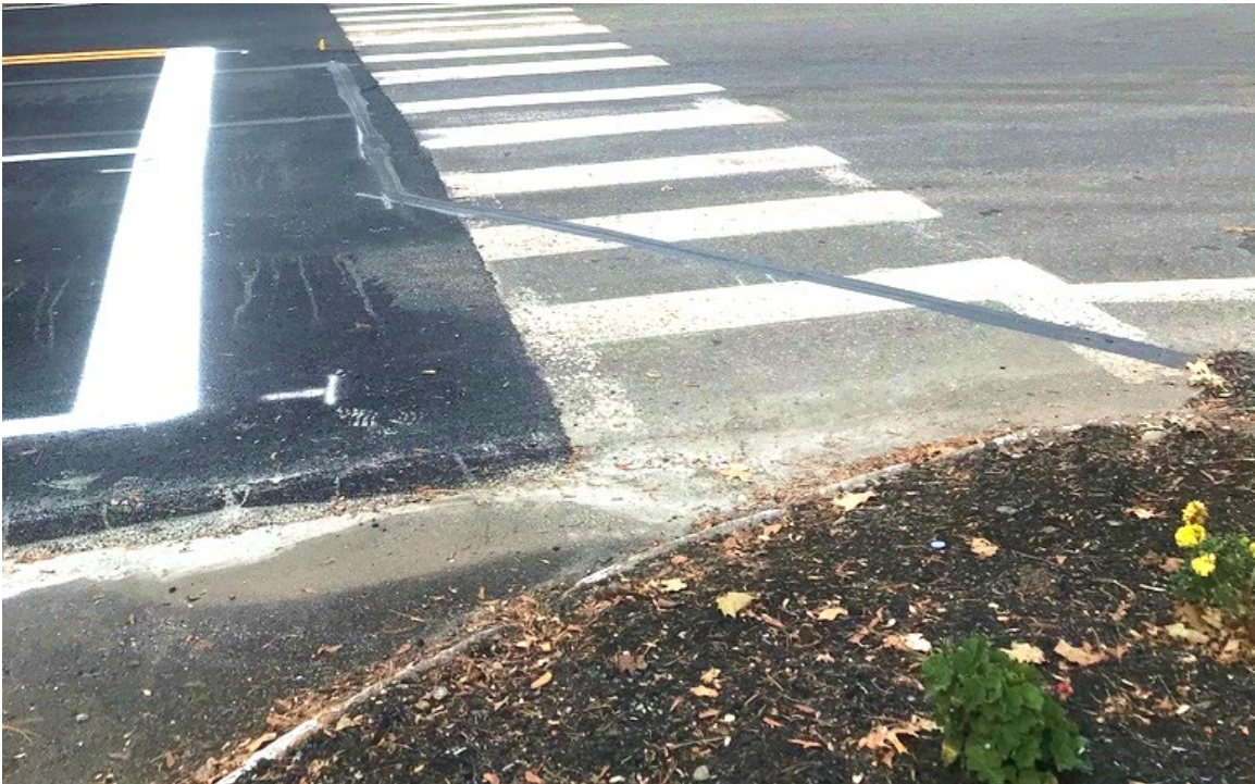
Figure 14 Lack of Pedestrian Facilities on Southwest Intersection Corner leading to Great Road (Route 117) Crosswalk
