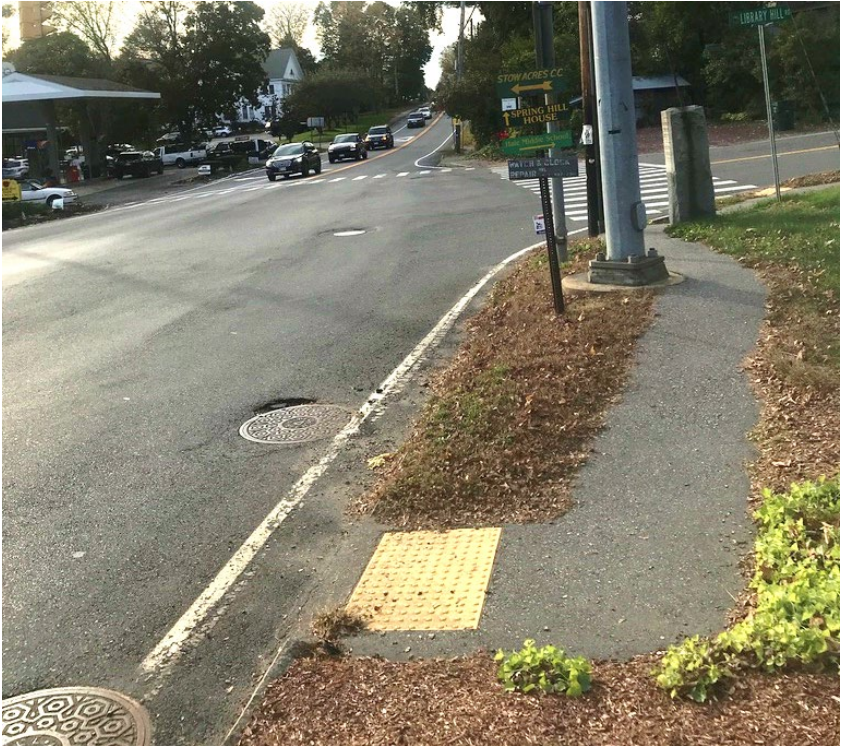
Figure 6 Great Road (Route 117 and 62) Crossing on Northeast Intersection Corner with Pedestrian Detectable Warning Strip Lacking Crosswalk
