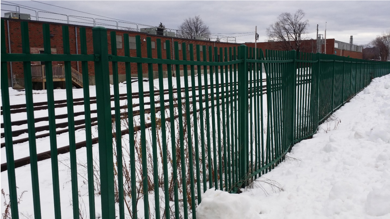
Steel fence damaged sections Belmont side.
