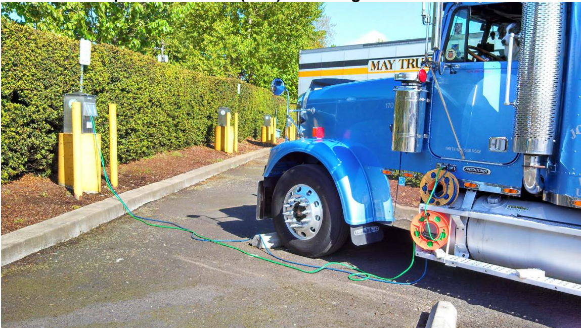
FIGURE 5 Truck Stop Electrification (TSE) Providing an Idle-Free Rest Break
